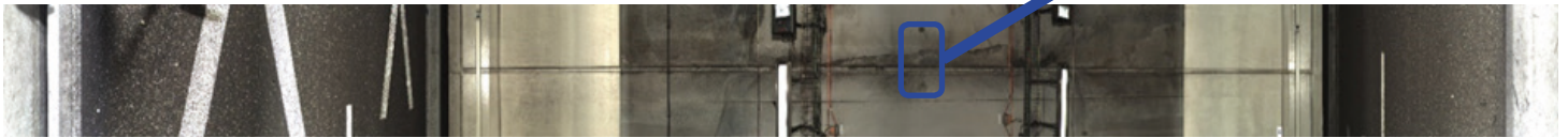
Panoramic of a tunnel section (diameter 12 m) – Zoom at the top of the vault
